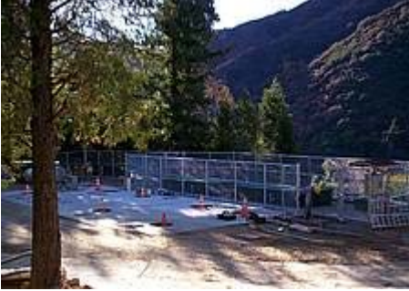
The new wastewater system included primary and secondary treatment.
